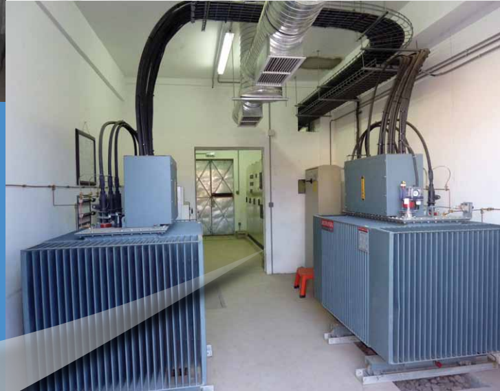
Poste de transformation 2x1000 KVA / Post of transformation 2 x1000 KVA
