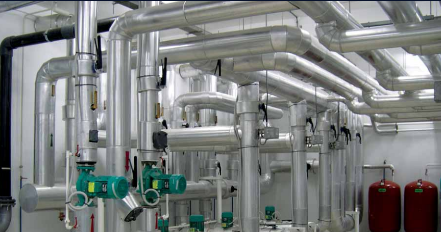
Chaufferie / Boiler room
