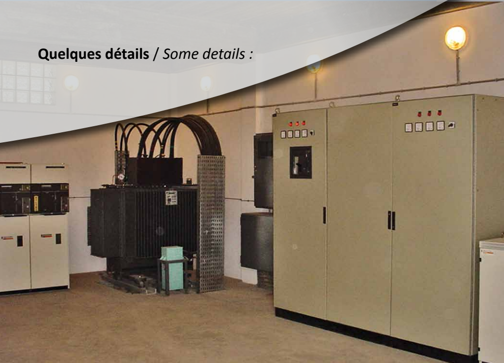
Armoire générale BT / LT general electric cupboard
